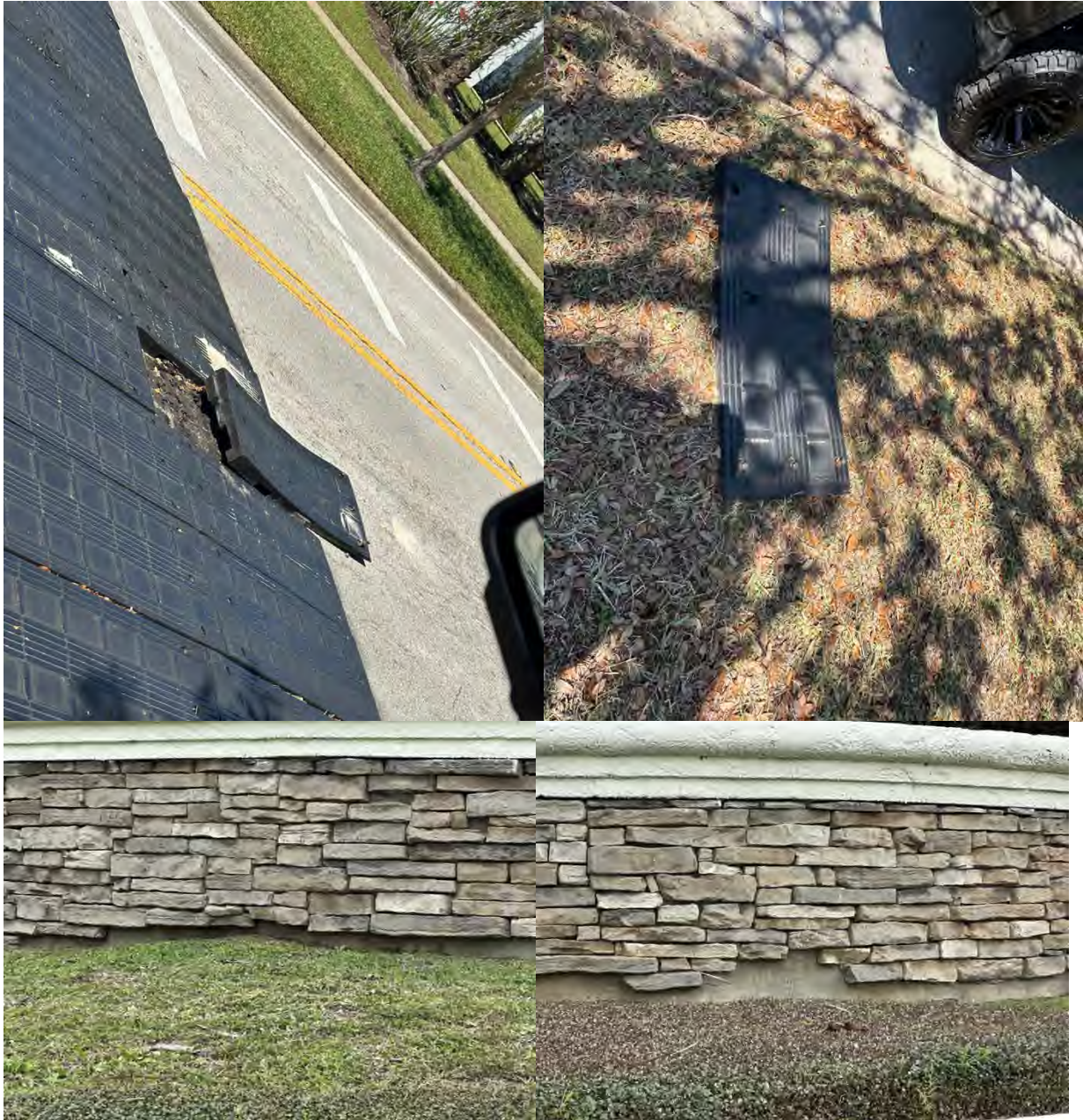
Stone facing falling off at entrance wall.
